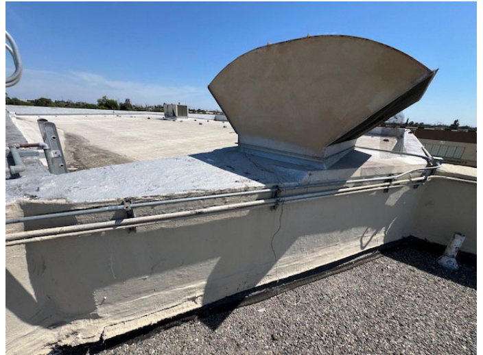
Silver Paint at Vent – Asbestos Containing
